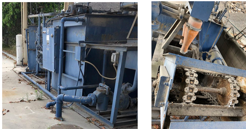
Original Bus Wash Equipment
