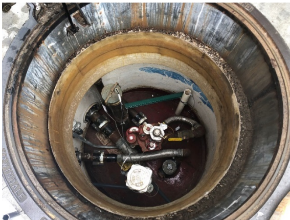
1.5 HP STP housed in tank-top sump
