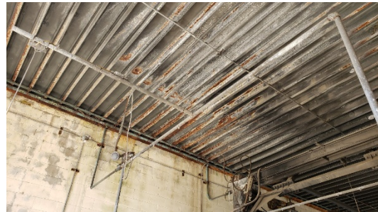
Figure S-12: Roof Metal Deck Corrosion
