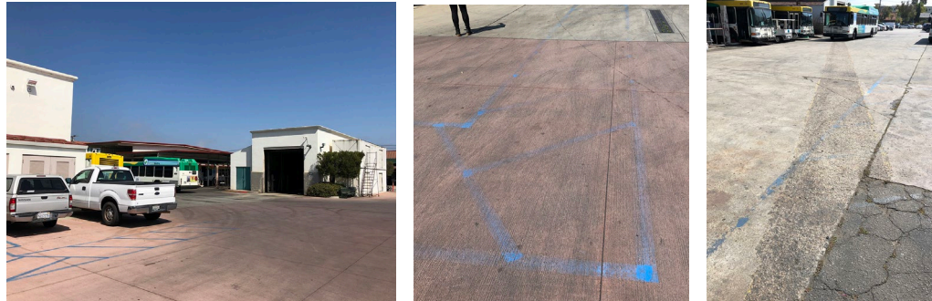
Worn Accessible Aisle Painting and Previous Accessible Aisle Painting, Since Removed
