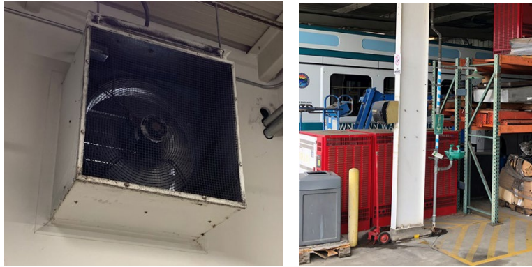
Electrical Room Wall Mounted Exhaust Fan / Eye Wash Station
