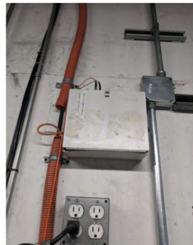
FIGURE F: WALL MOUNTED TELECOMMUNICATIONS ENCLOSURE IN SOUTHEAST ELECTRICAL ROOM
