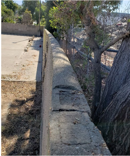
Figure S-15: Masonry Wall Buckling
