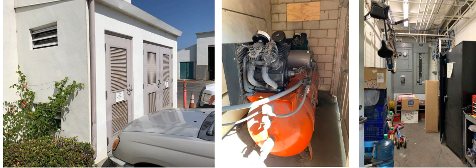
Air Compressor Enclosure / Air Compressor / Electrical Room
