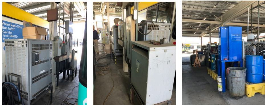
Aisle 4: Old E-bus Chargers between Aisles 4 and 5 / Misc. Equipment and Used Fluids
