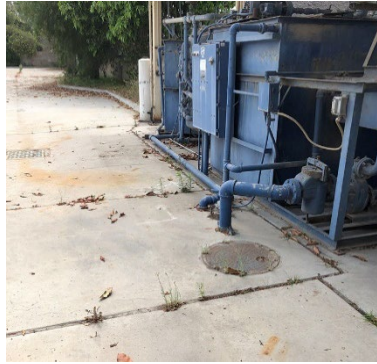
Bus Wash Equipment & Sump Pit
