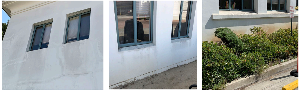
Cracking in the Plaster Veneer / Water Staining Under Window / Staining of Plaster Finish Behind Landscape
