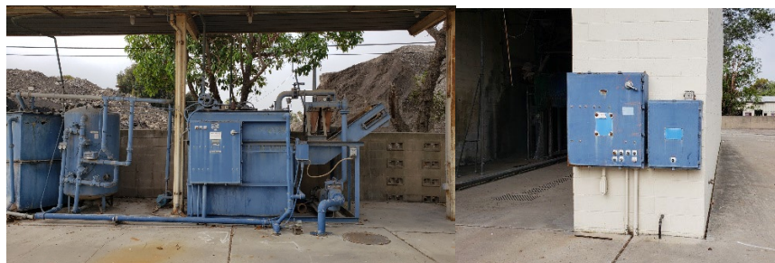
Electrical Panels CP-1 & CP-2
