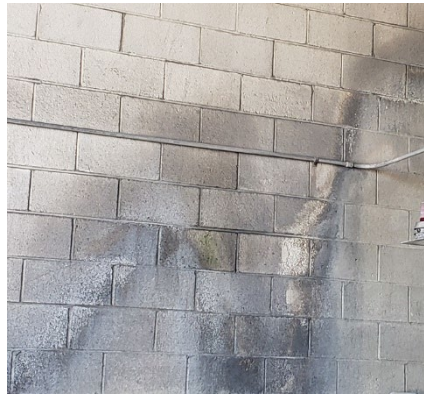
Figure S-7: Masonry Water Staining
