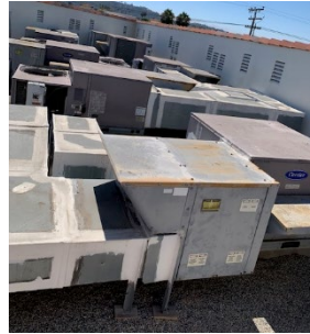
Figure 3: Properly Maintained Ducting
