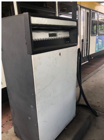
Gasboy Dispenser at East Service Island
