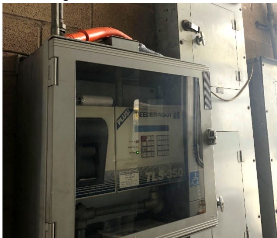
Leak Monitoring Console Located in Utility Tower
