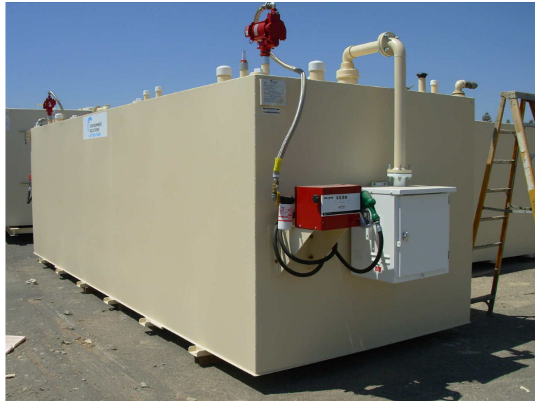
Example of Temporary AST
