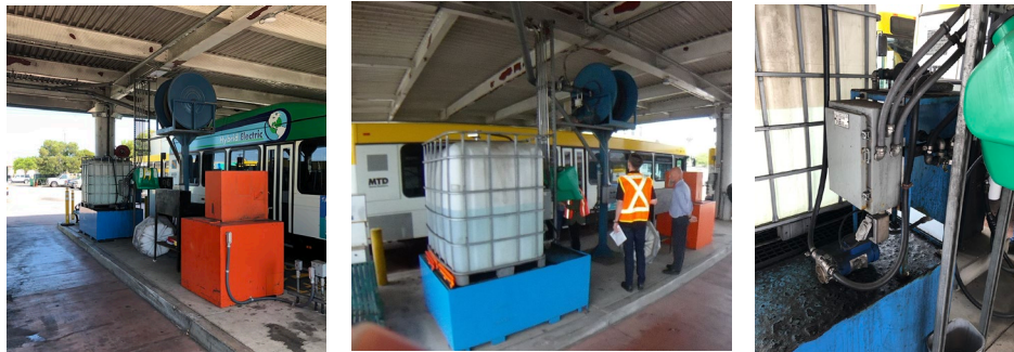
Center Island: Fare Vault, Vacuum System, and DEF Tank
