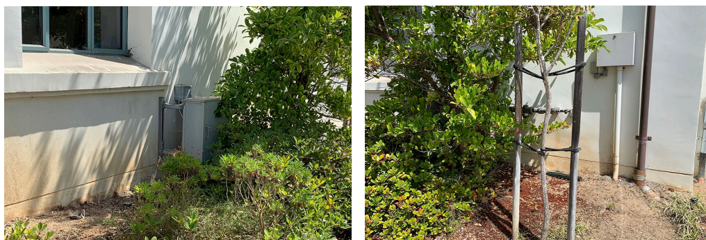
Utilities Hidden Behind Vegetation
