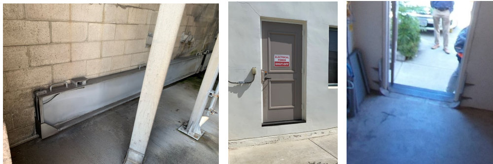
Flood Stop Barriers Stored in Wash Bay / Entry to Electrical Room (110) is Elevated +12" from Exterior Grade / Flood Stop Threshold Within Room
