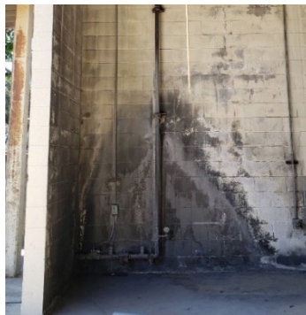
Figure S-11: Water Staining
