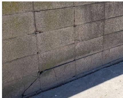
Figure S-17: South Wall Cracking
