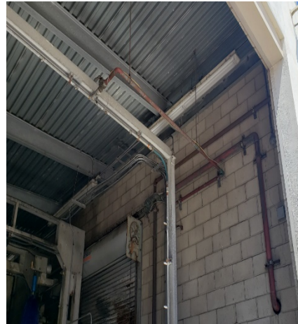
Figure 21: Wash Bay Piping
