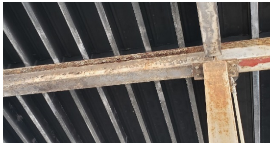
Figure S-10: Beam Rust and Paint Peeling
