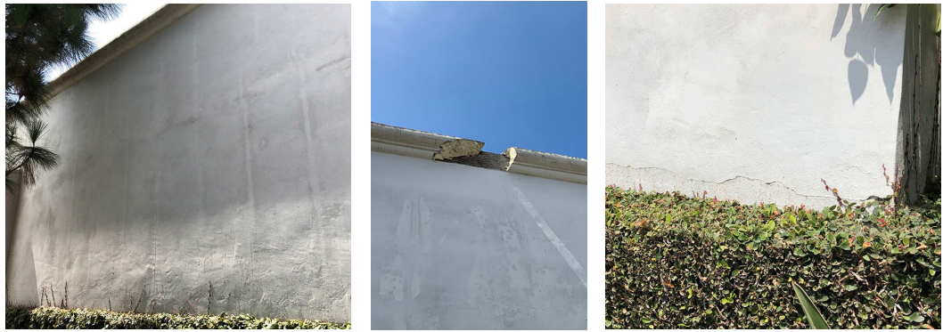
Metal Framing Outline Through Plaster / Broken Parapet Cornice / Crack at CMU Transition
