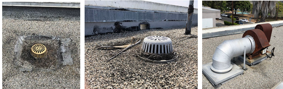
Maintenance Building Roof Drains / Roof-top Exhaust Fan
