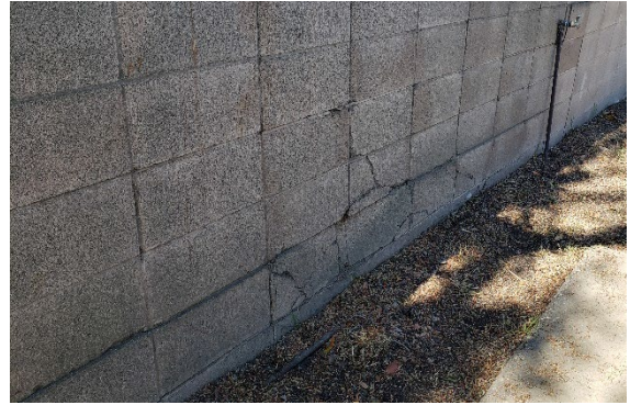
Figure S-16: South Wall Cracking
