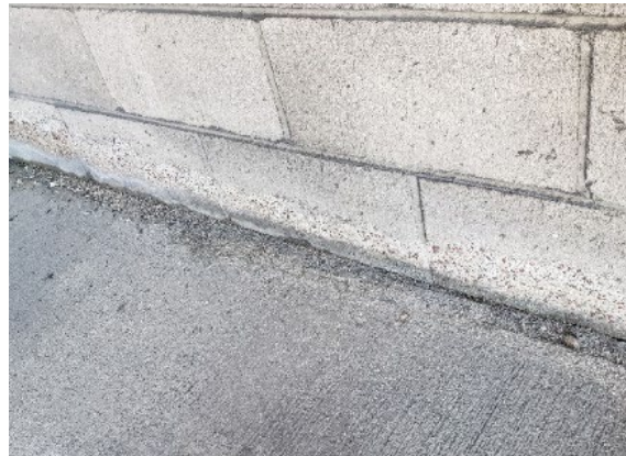
Figure S-7: Concrete Masonry Erosion
