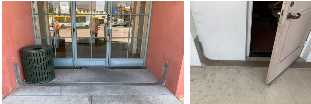
Flood Stop Threshold at Staff Entry (115) Door / CAD Dispatch (104) Exterior Door
