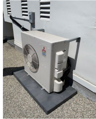
Figure 2: Mitsubishi Split System Units
