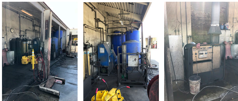
Mobile Lift Used for Chassis Wash / Wash Bay Equipment / Hot Pressure Washer
