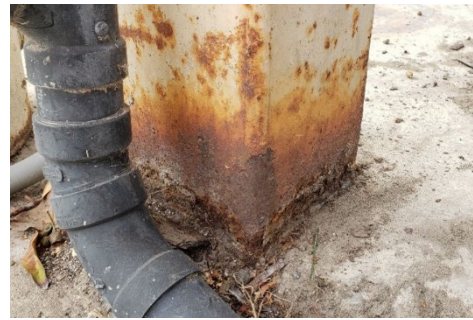
Figure S-14: Canopy Column Base Deterioration
