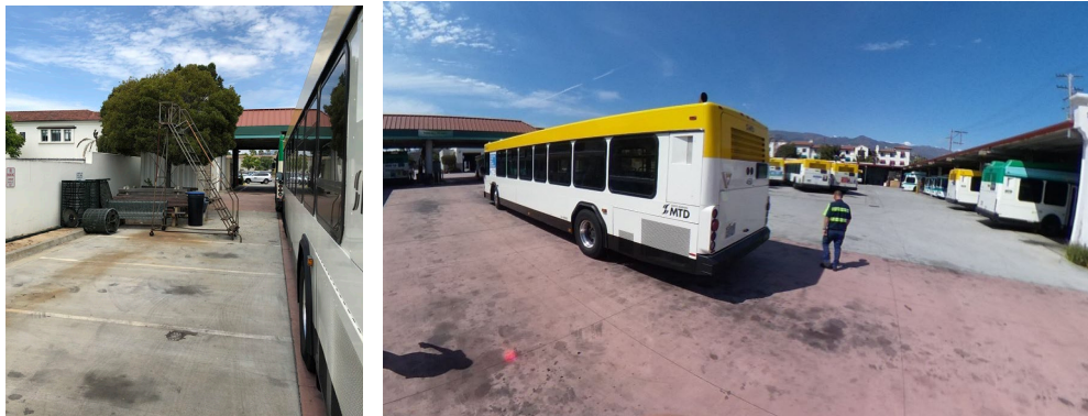
Staining at Parking and Queuing Areas South of Fuel Island
