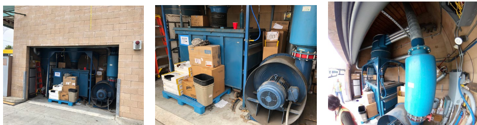
Utility Tower and Vacuum System
