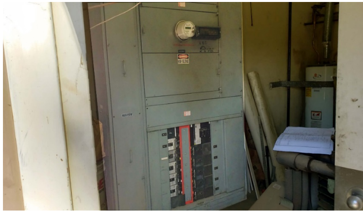
Main Distribution Board
