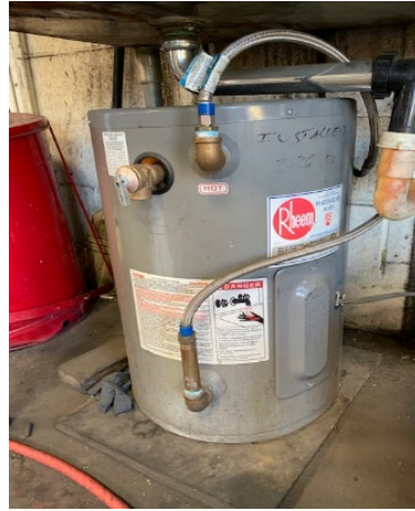
Figure 16: Rheem Water Heater
