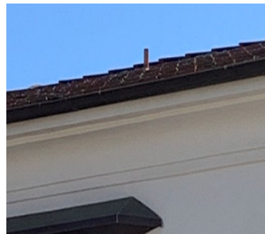
Figure 8: Properly Ventilated Bathrooms
