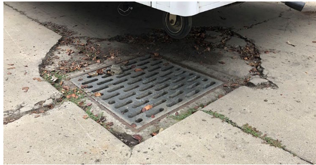
Failing Pavement at Catch Basin
