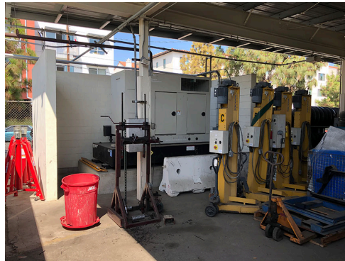
Generator at North Corner of Canopy
