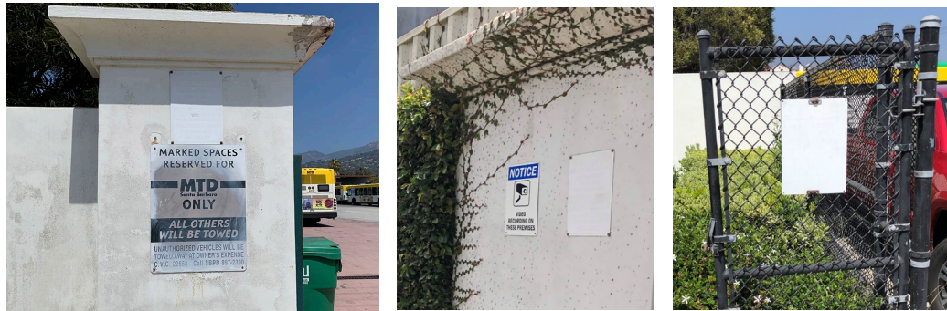
Weathered and Missing Perimeter Signage
