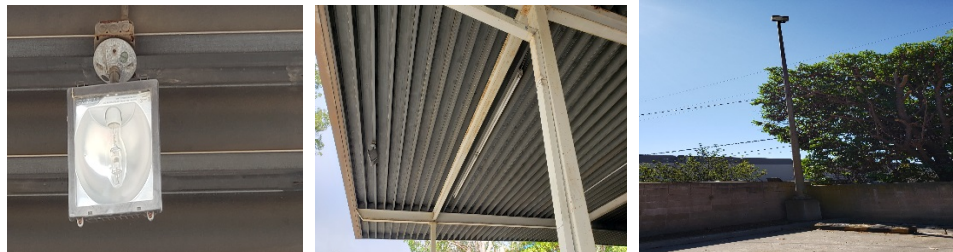
Floodlights / Fluorescent Strip Lights / Pole Mounted Flood Lights
