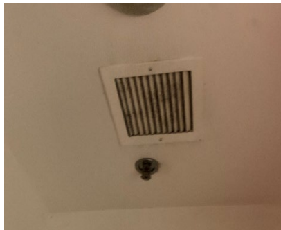
Figure 7: Ceiling Exhaust Grille
