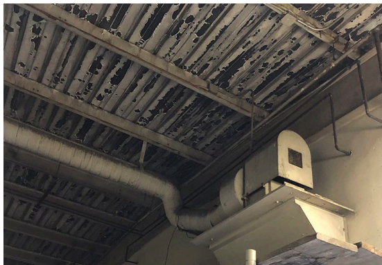
Peeling Paint and Tailpipe Exhaust Fan with Ductwork
