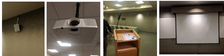
Auditorium A/V System
