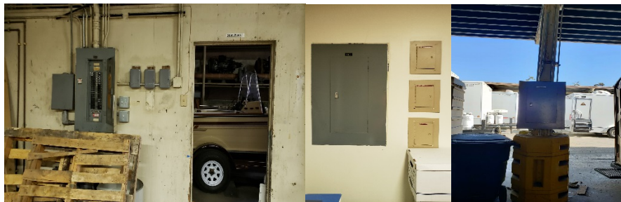
Electrical Panels A, B & D
