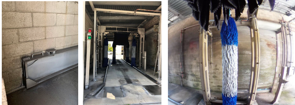
Interior of Bus Wash: Admin Bldg. Flood Plate / Wash Equipment / Rusted Coiling Door
