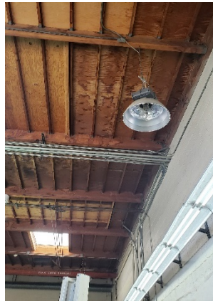
Figure S-2: New Framing and Water Damage
