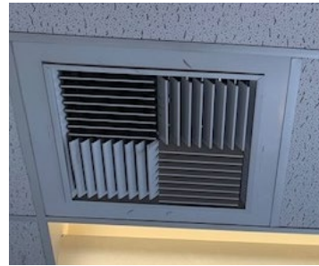
Figure 4: 24"x24" Diffusers (Typical)
