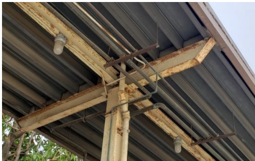
Figure S-13: Rusty Canopy Steel Beams and Columns
